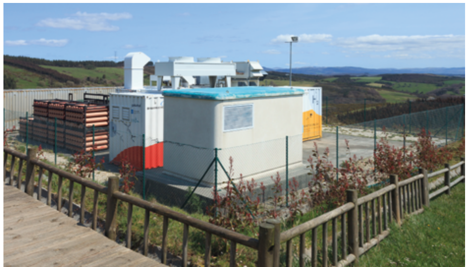
Hydrogen production facility using electricity generated by the Sotavento wind farm in Galicia (Spain) [1].
