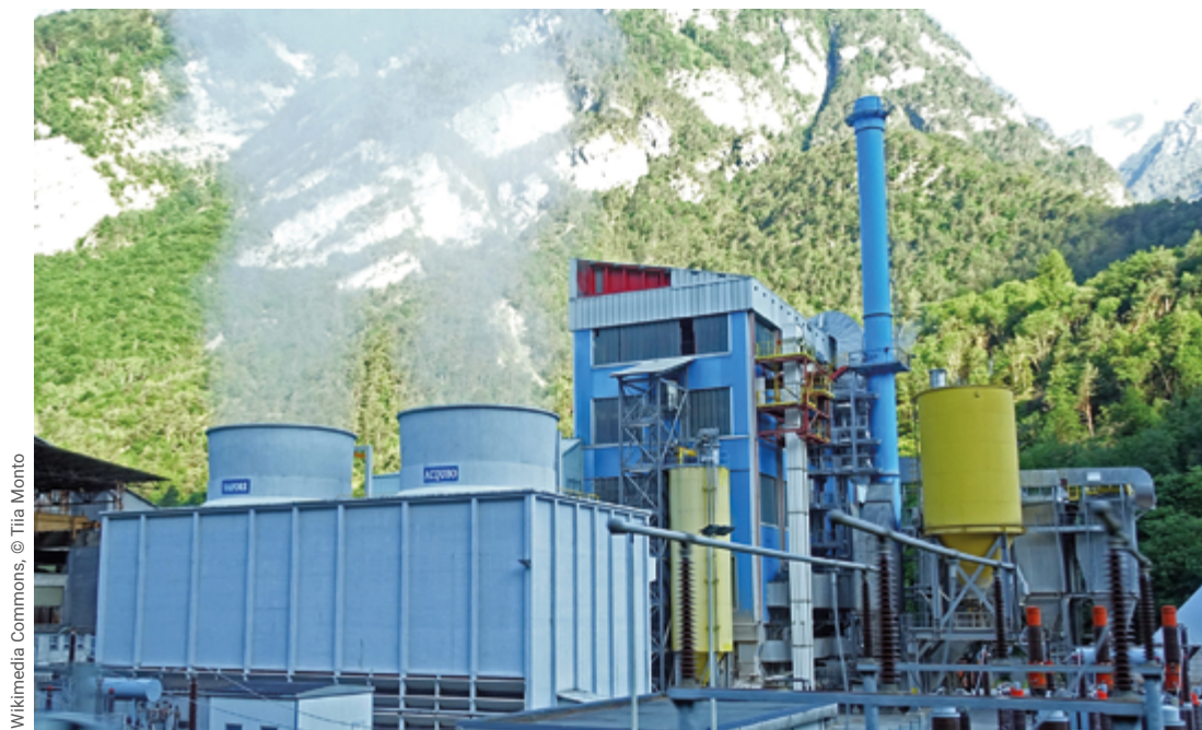
SICET, a biomass power plant in Ospitale di Cadore, in the Veneto mountains in Italy. The plant generates electricity using the steam released by the combustion of plant matter, which drives a turbine connected to an alternator.
